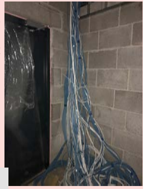
Server room at HoH on May 21st, 2019.
